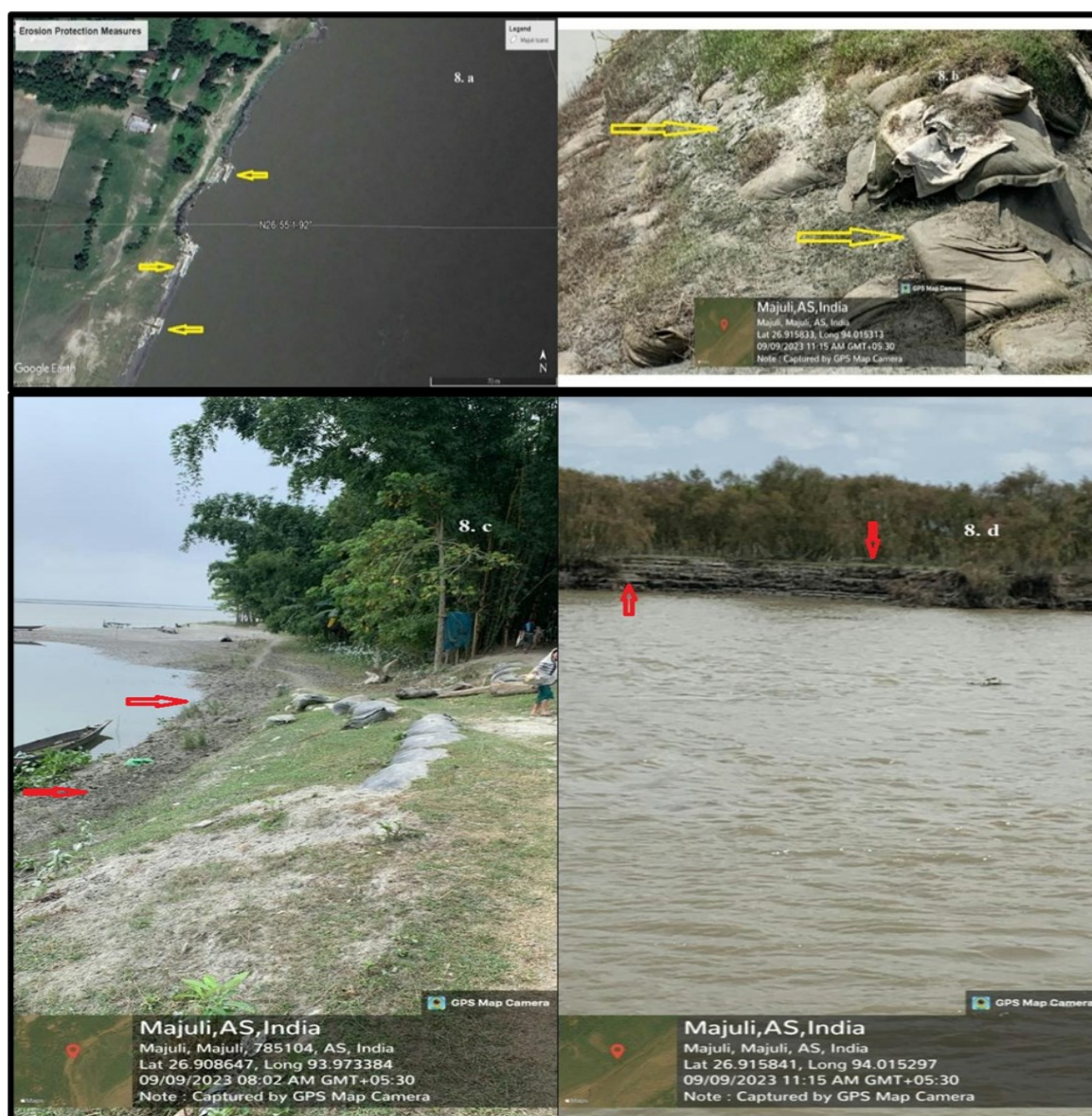
Fig. 8. (a) Satellite image of embankments on riverbank; (b) Damage of embankments due to severe erosion; (c) Severe soil erosional site; (d) Riverbank protection measures
