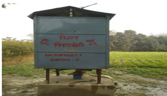
Fig. 1. Tube well with pumping Shed unit.
