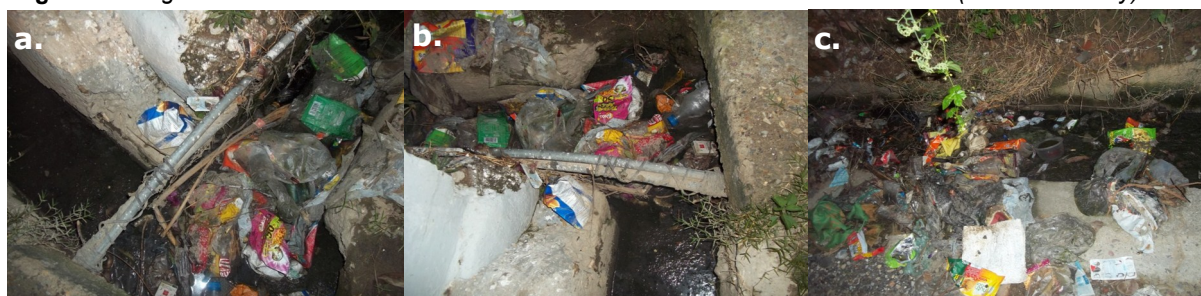
Fig. 3 (a-c). Water supply pipes passing through drains at the old Jammu distribution point.
